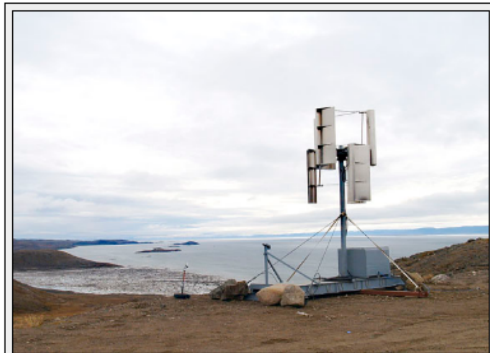
A vertical turbine windmill spins outside the Arctic Winter Games arena in Iqaluit Sept. 23. Nunaworks of Iqaluit hopes to begin manufacturing and selling the windmill within Nunavut. (PHOTO BY CHRIS WINDEYER)
